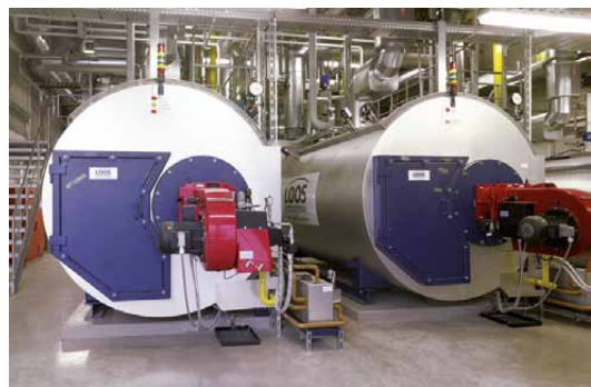
Steam consumption is also monitored
